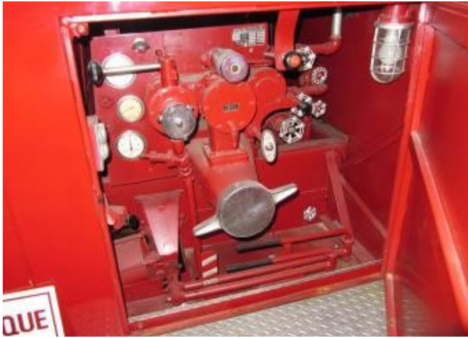
The various gauges and valves of the pump panel
